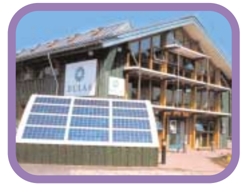
1.4kW photovoltaic array supplying about 10% of the annual electricity demands of the offices of Dulas Ltd, Machynlleth
